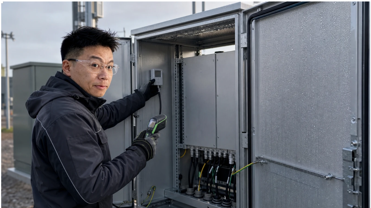
Why Outdoor Telecom Cabinets Condense—and How to Prevent It
