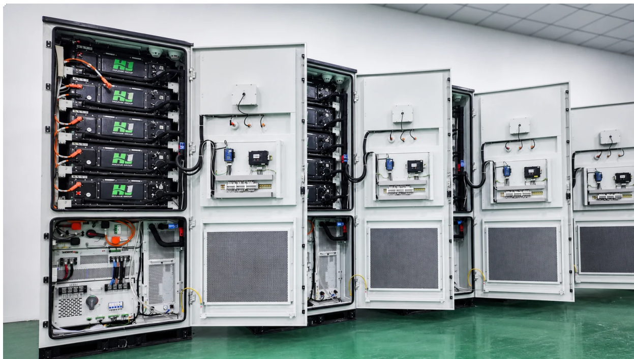
Solar Charge Controller vs Telecom Rectifier in a Hybrid Site
