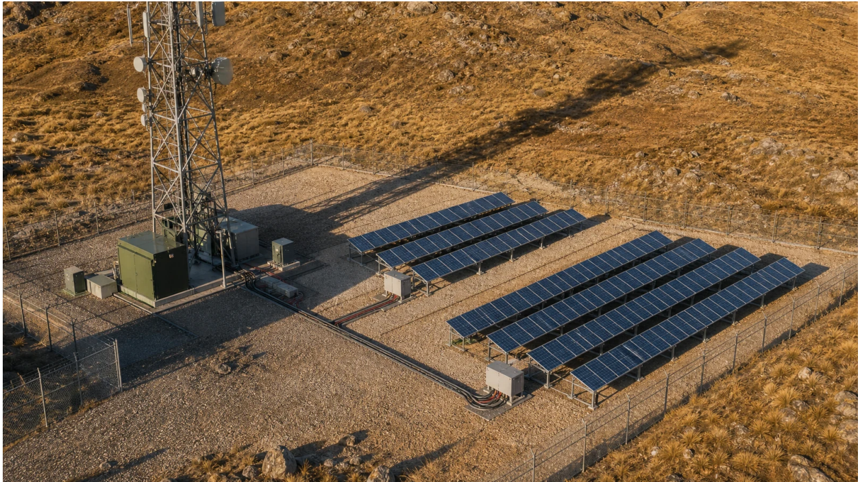
Solar Panels for Telecom Towers: Voc, String Design and Shading Checks
