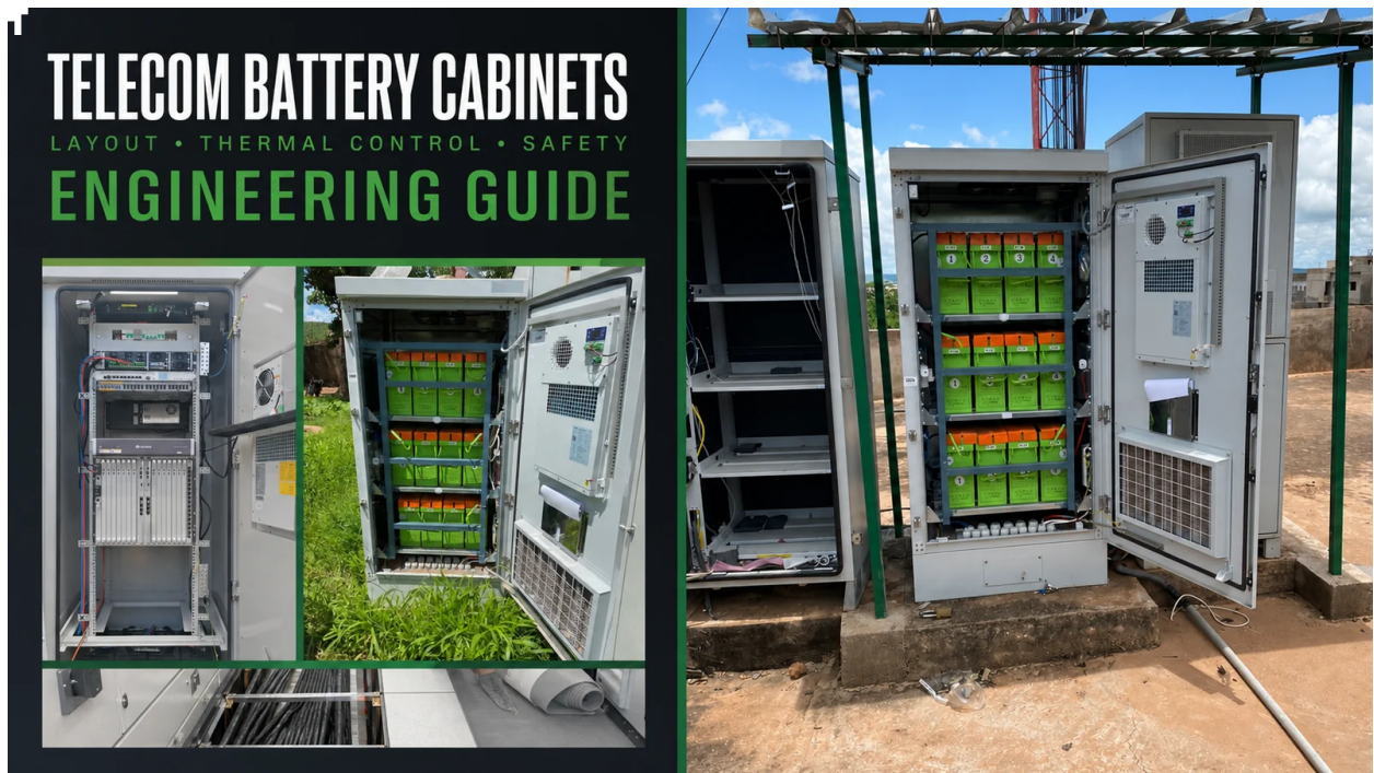
Telecom Battery Cabinets: Layout, Thermal Management and Safety
