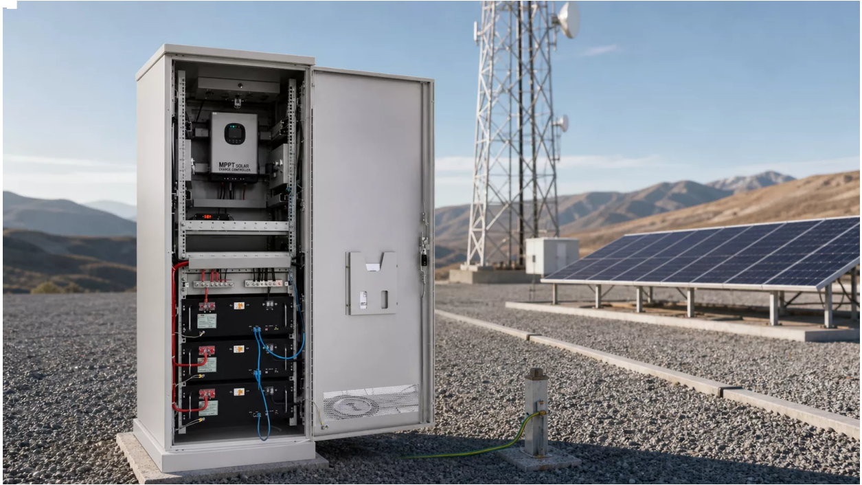
Integrated Telecom Energy Cabinet: Components, Architecture and Selection Guide
