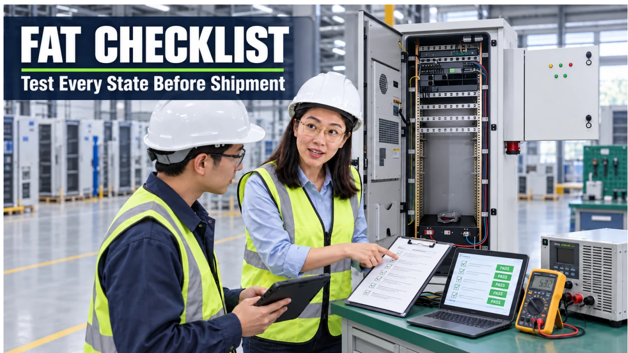
Telecom Power System FAT Checklist: What to Test Before Shipment
